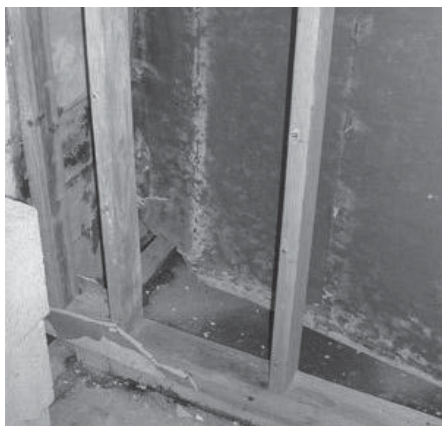
Mold inside a wall cavity
