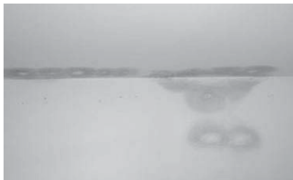
Water stains on drywall
