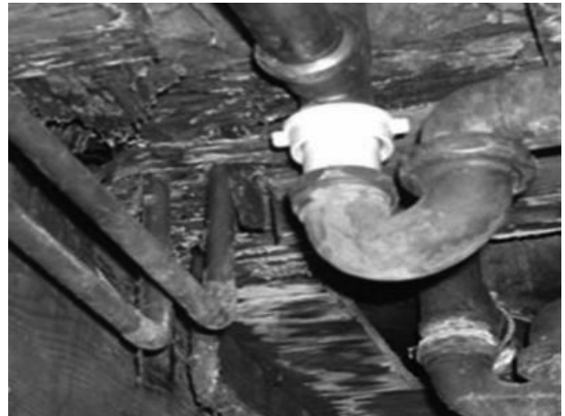
Mold growth because of bathtub leak
