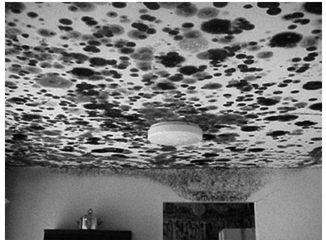
No testing to verify mold, needed here
