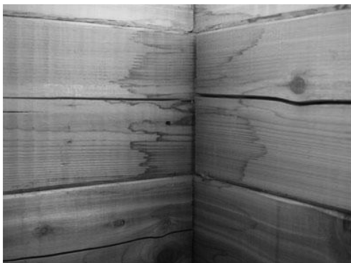
Permanent water stains on wood
