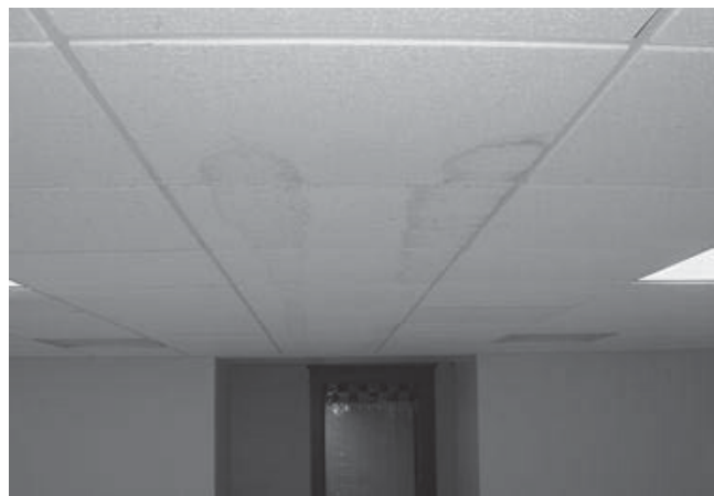
Water stained ceiling tile
