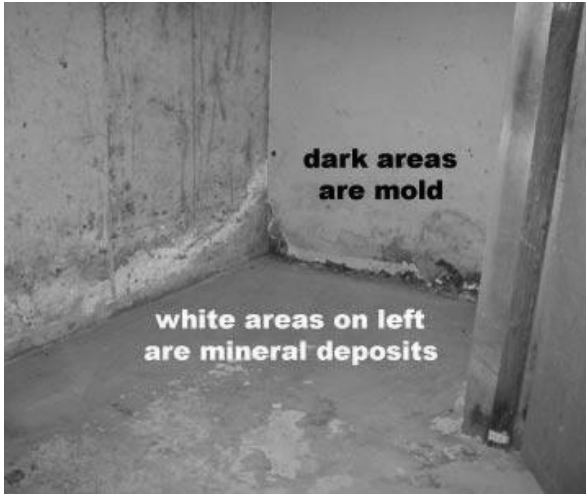
Water penetrating through foundation walls
