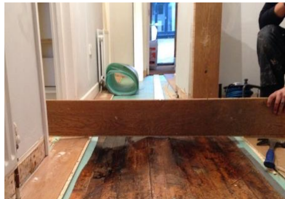
Buckling of Floor Above
