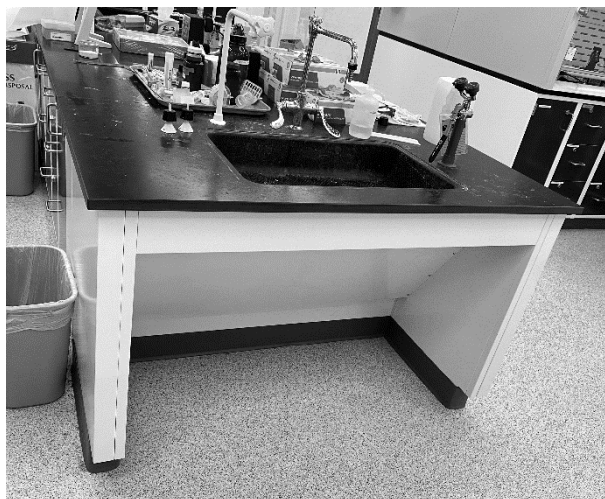
Accessible Sink and Eye Wash
