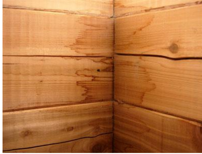
Permanent water stains on wood
