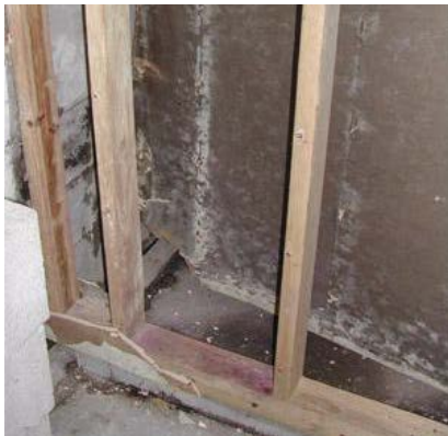
Mold inside a wall cavity
