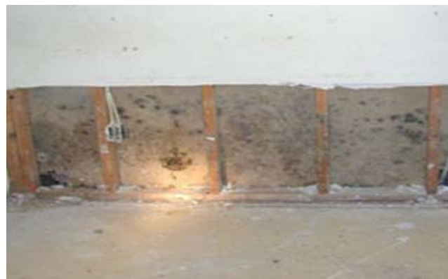
Mold on the back side of drywall
