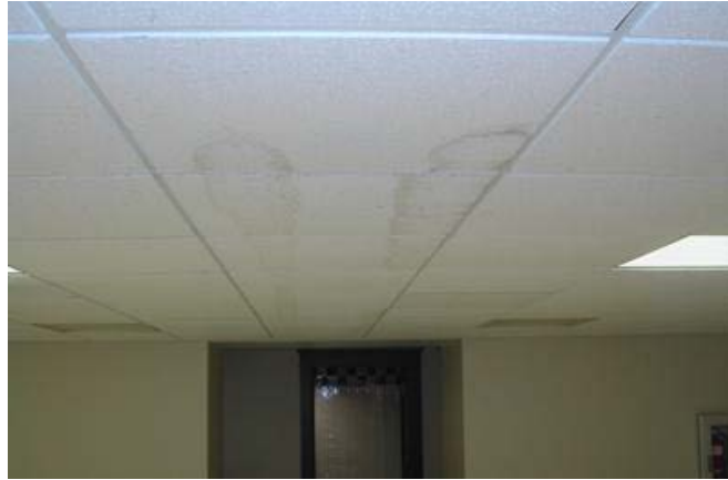
Water stained ceiling tile
