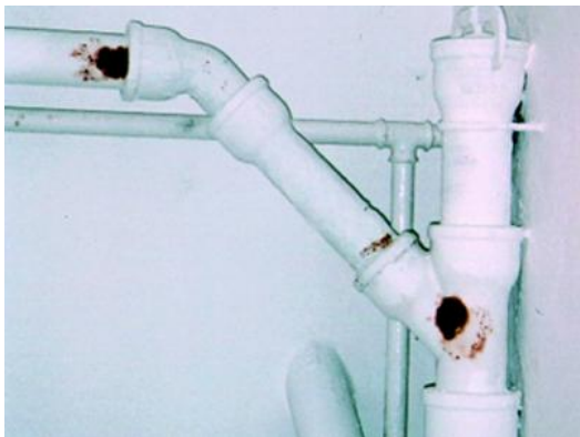
Evidence of leaky pipe joints
