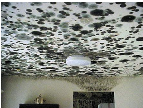
No testing to verify mold, needed here
