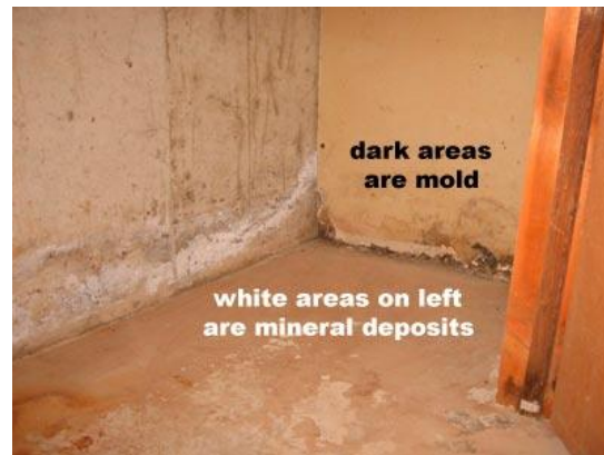
Water penetrating through foundation walls
