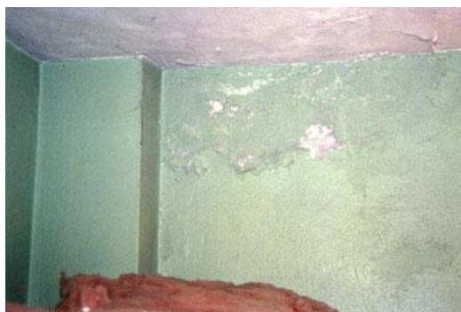
Roof leak affecting the wall below
