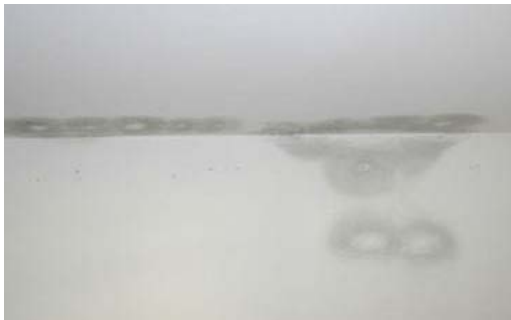
Water stains on drywall
