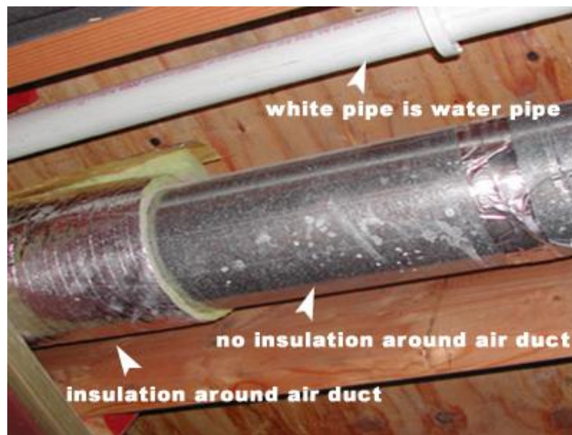
Condensation on air duct
