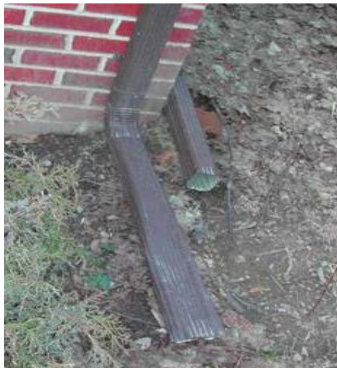
Settling because drainage systems not maintained
