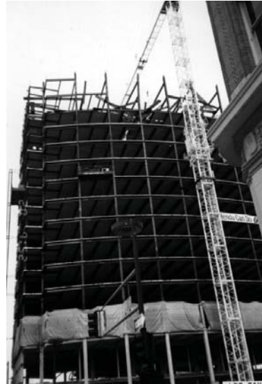
Construction of a modern steel frame building in which the ends of beams are rigidly joined to columns by welded connections.
